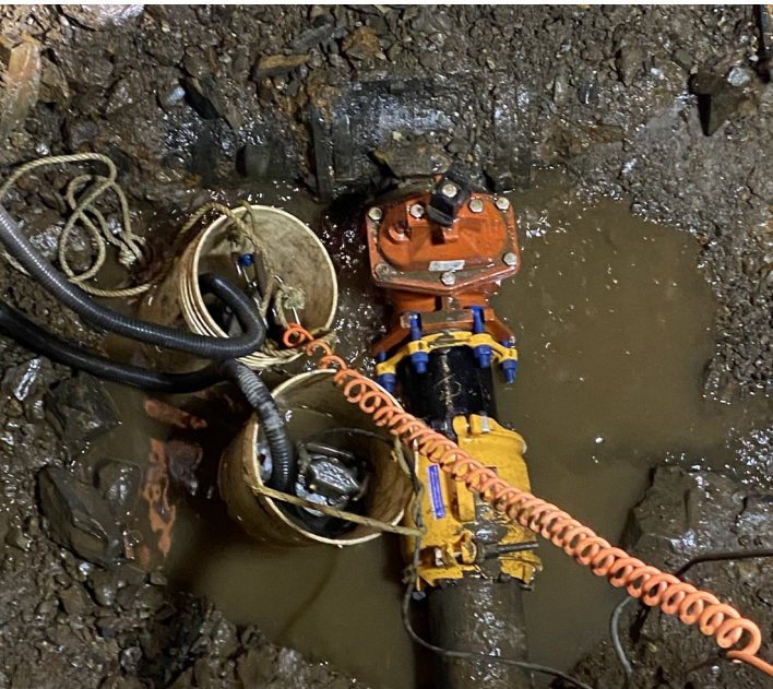
On Monday the 15th, the standby person received a call to shut off the domestic and fire service for the Sunrise Motel due to a leak.
