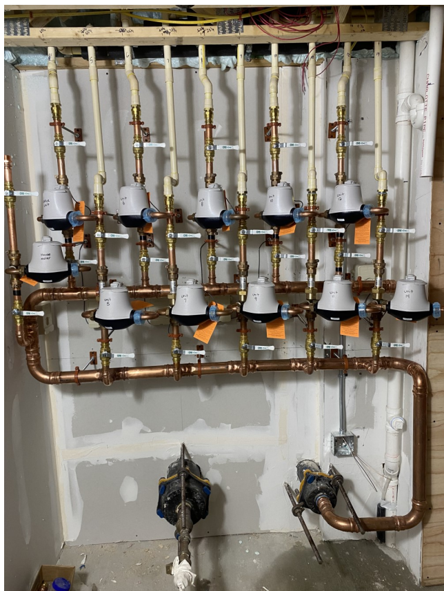
11 new meters for a combined commercial & residential project
