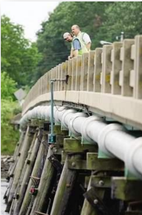
Don Neumann and Todd Hill show how the existing water line along the Route 103 bridge will be moved about 60 feet under the river.
