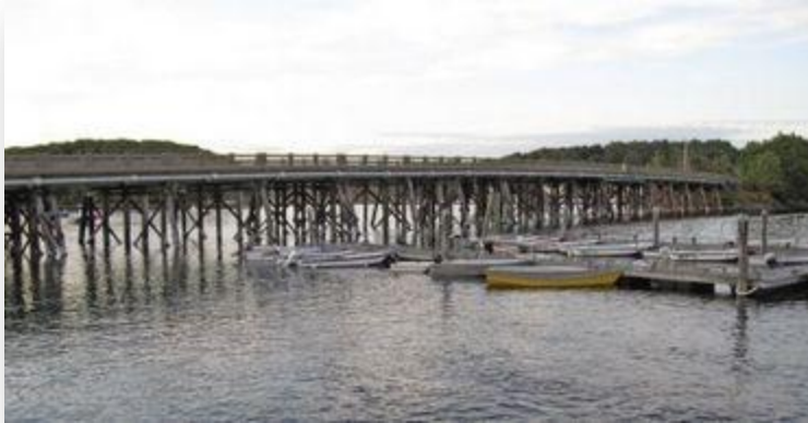
The Route 103 bridge over the York River was closed by the state Tuesday for renovations.
